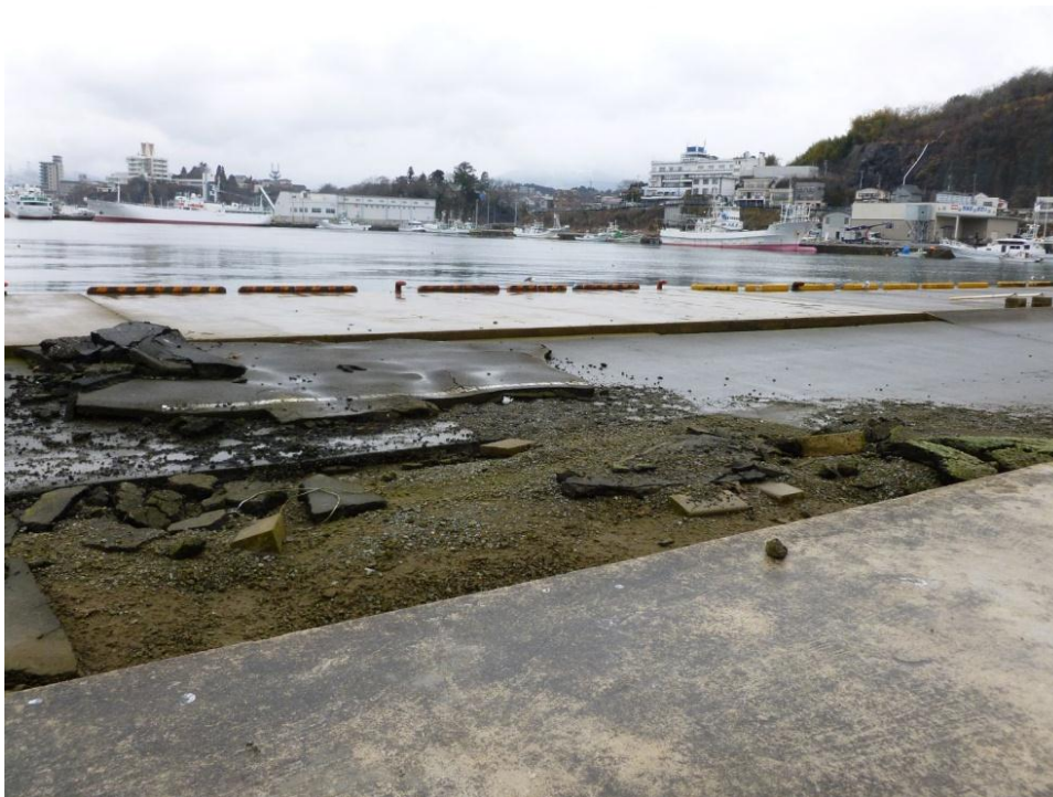
Figure VII.2. Pile-supported dock with local subsidence failure of dockside infill: Kesenuma Port, Japan, March 10, 2012, one year after tsunami.
